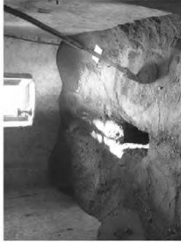
TRADITIONAL LADAKHI IRRIGATION CHANNEL SYSTEM
